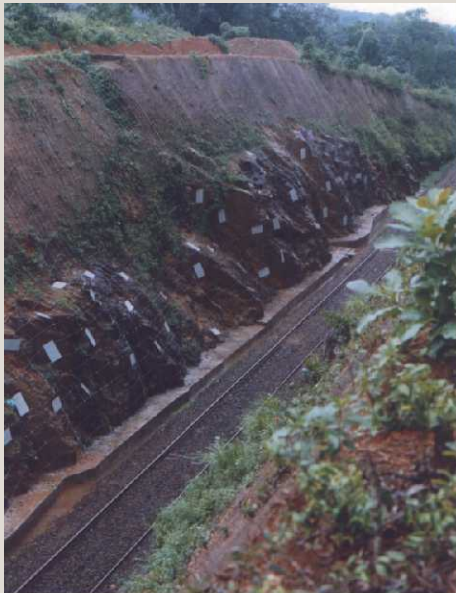
Steel wire ropenet at Southern Railway
