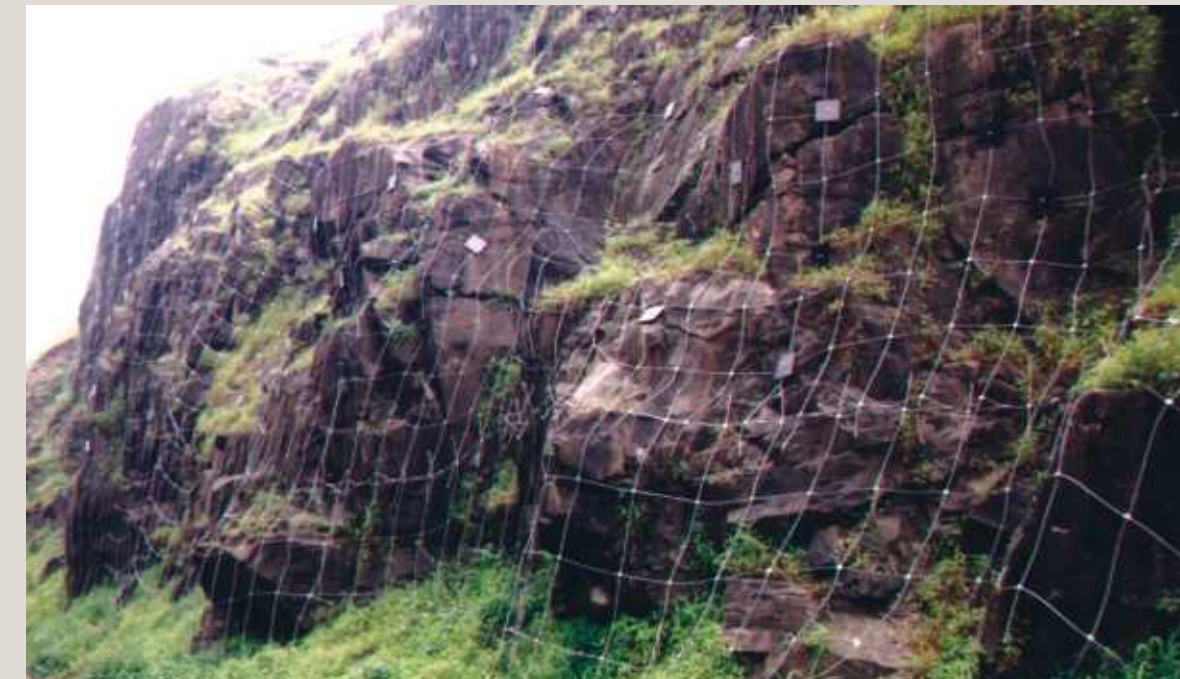
Steel wire ropenet at Bijghar Cutting, KRCL
