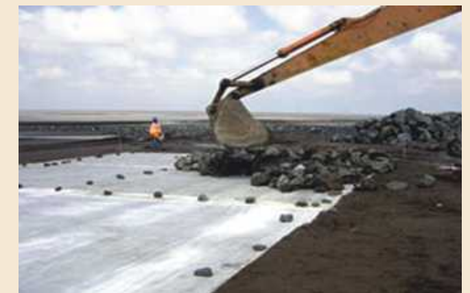
Filter cum separator at L&T Shell Hazira site
