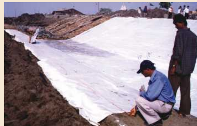
Geotextile filter below erosion control bund at Moti Danti, Valsad
